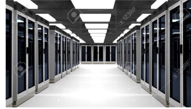
Datacenter: Fans, Lighting, Servers, Mining Devices
